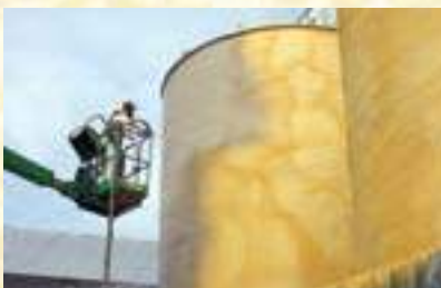
Insulation for industrial storage tank
